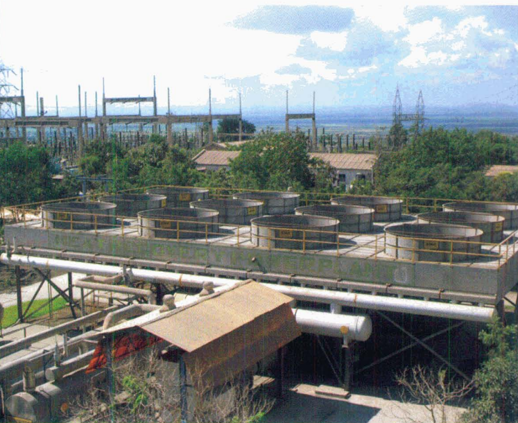
The waste heat recovery system at Andhra Pradesh Cement works.
